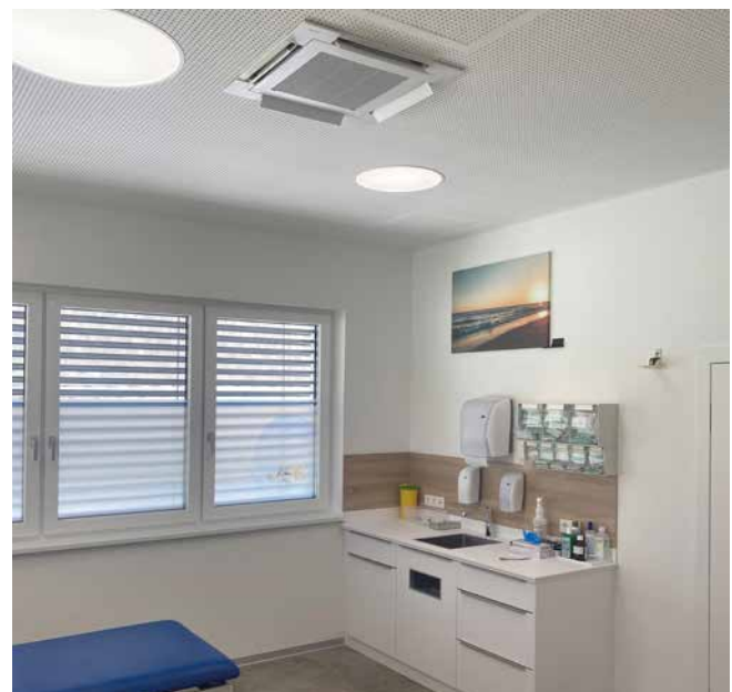
Ordination Groß St. Florian, Cool Company Kälte - Klima - Gastro
